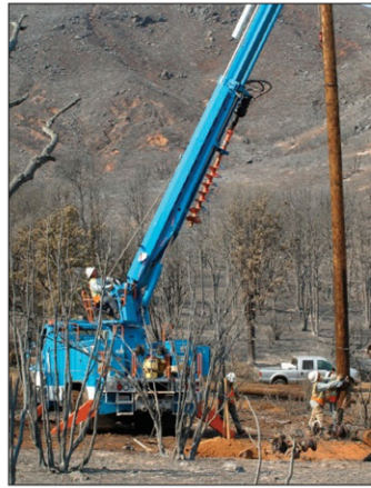
Pacific Gas & Electric Co.
